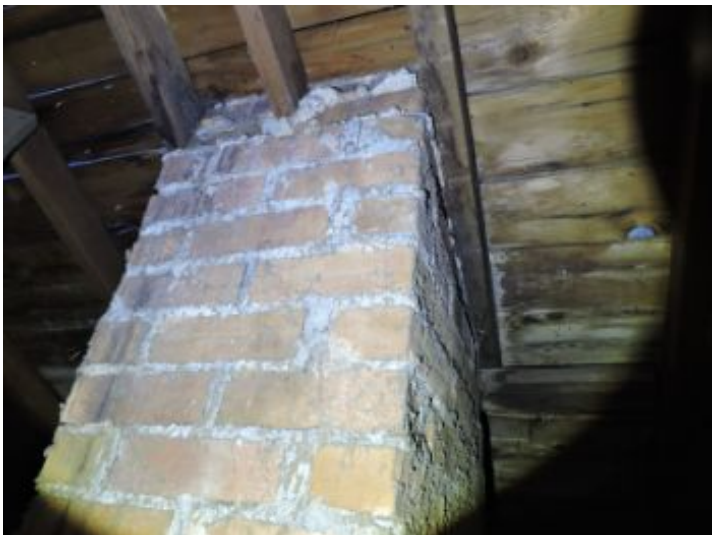
Example view - chimney/stains from prior leaks
