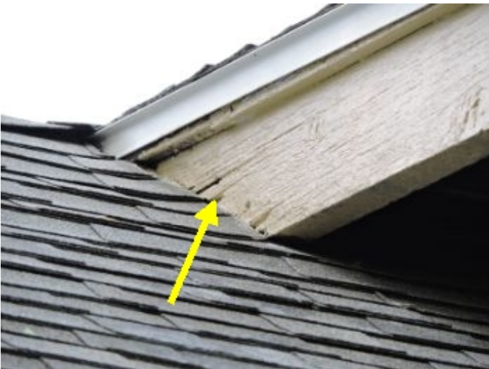
Example view - worn paint/possible decay at wood fascia - SW
