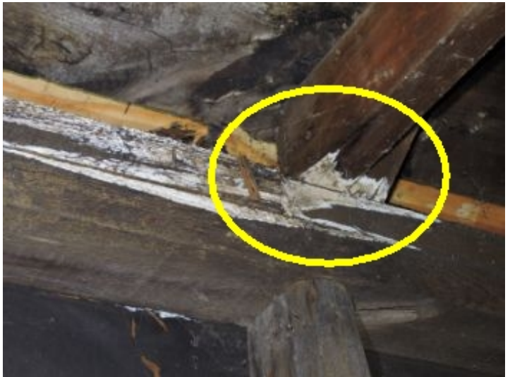
Example view -decay at walls/rafters - garage
