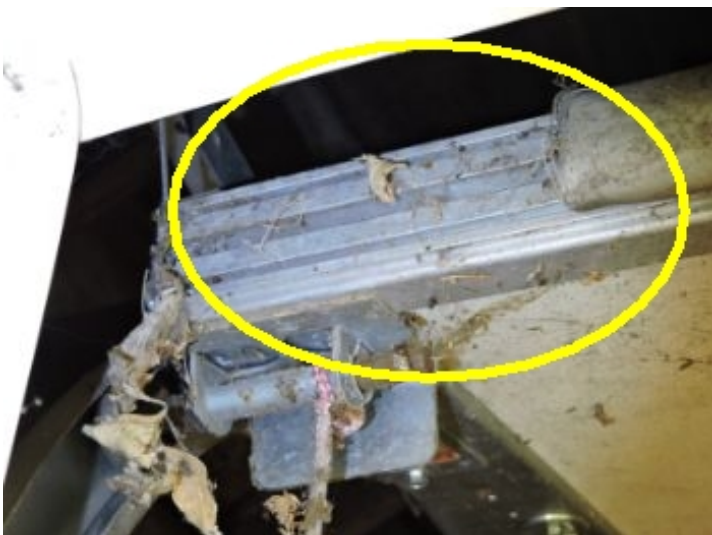
Example view - damaged weather stripping - garage door
