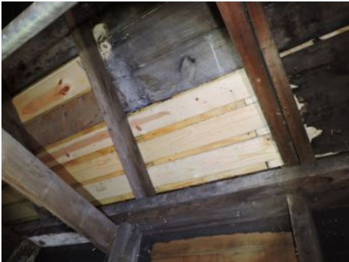
Example view - prior repairs to board sheathing - garage
