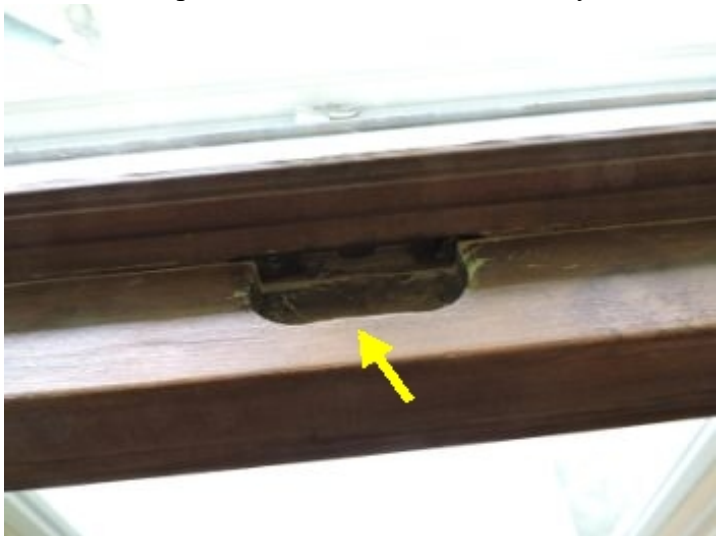
Example view - missing/damaged latch hardware - bathroom window - north
