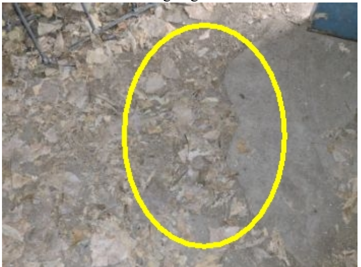
Example view - cracked/damaged floor - garage
