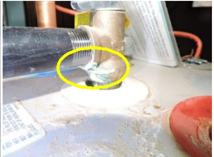
Example view - corrosion at TPR valve - water heater
