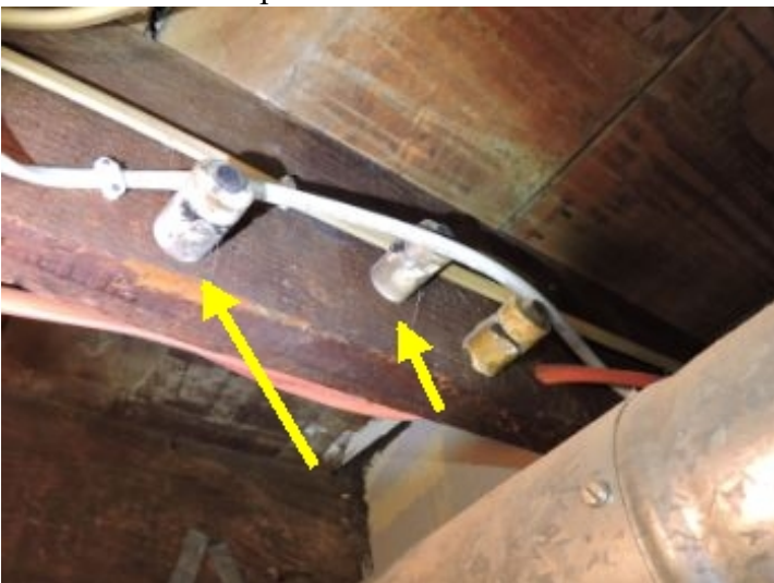
Example view - abandoned knob and tube electrical - basement
