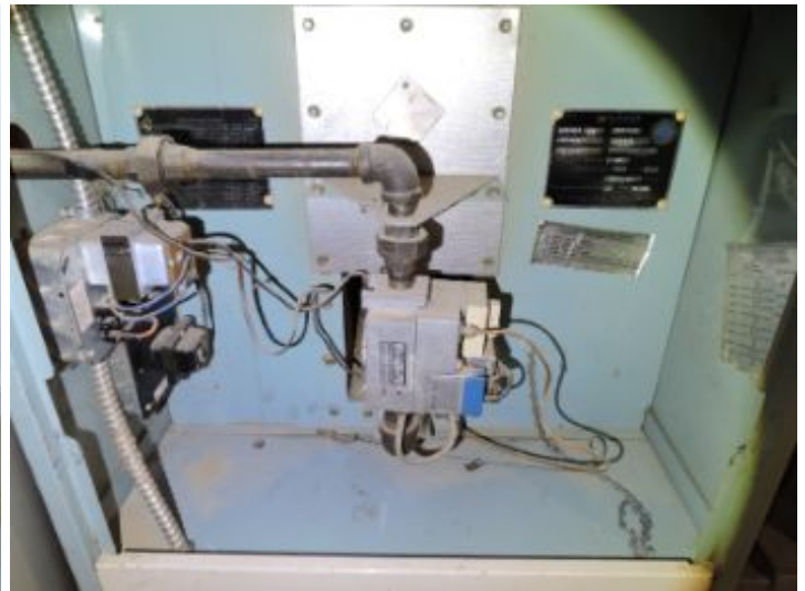
Example view - interior of furnace cabinet
