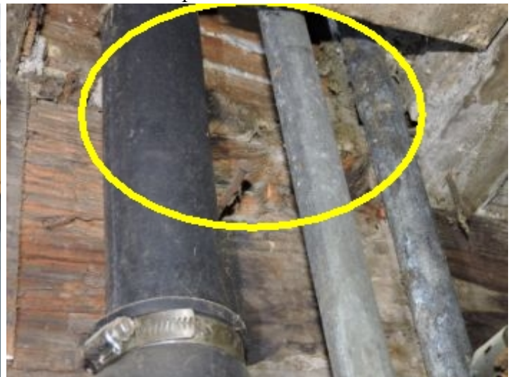
Example view - decay at joists - basement
