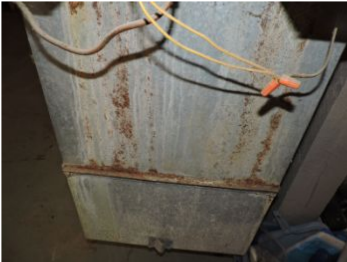
Example view - rust/corrosion at forced air ducts under humidifer
