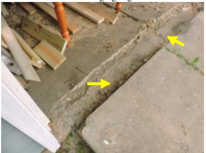
Example view - damaged/settled concrete floor - garage driveway
