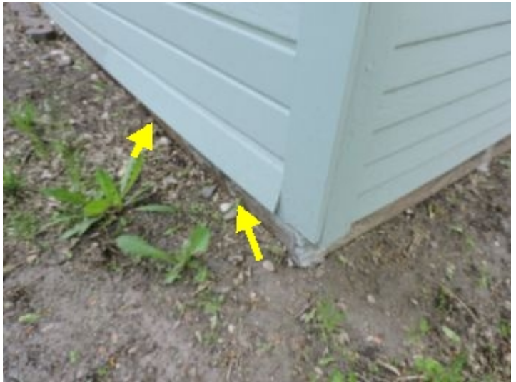
Example view - bulge at east side of garage siding
