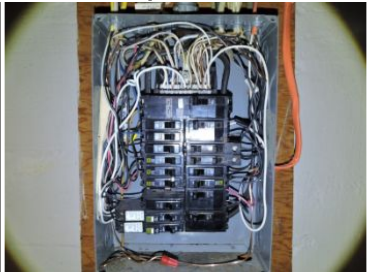
Example view - interior of main electrical panel
