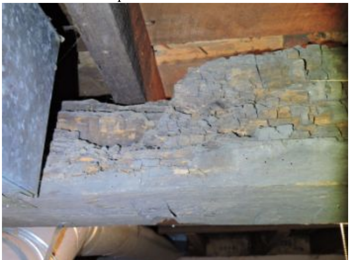
Example view - decay/damage to main support beam - basement
