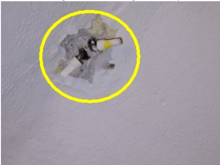
Example view - improperly terminated electrical wires - NW bedroom closet
