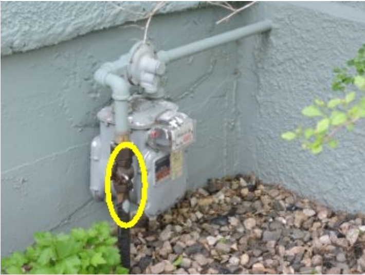
Example view - gas meter/main shut off valve
