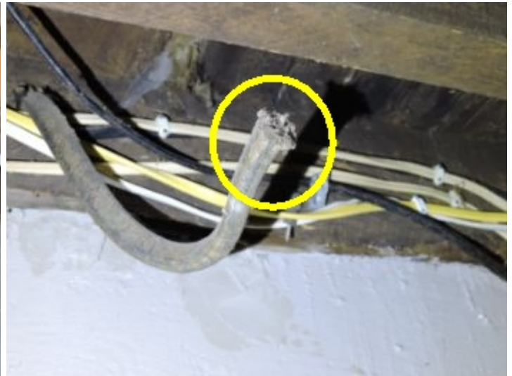
Example view - improperly terminated electrical wire - basement above main panel
