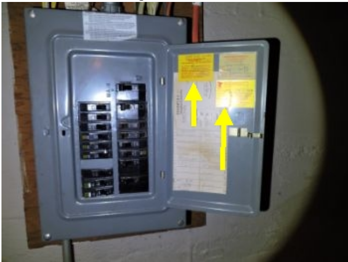
Example view - main electrical panel /MN state electrical inspection stickers
