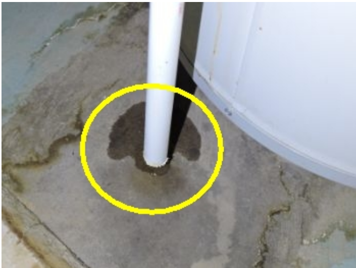
Example view - water discharge from water heater
