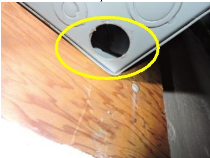
Example view- missing knockout - main electrical panel
