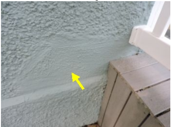
Example view - evidence of prior repairs to stucco
