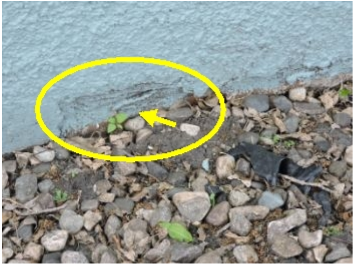
Example view - damage to foundation protective covering
