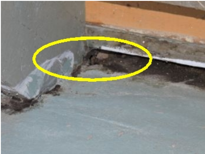
Example view - decay at basement stair stringer(s)
