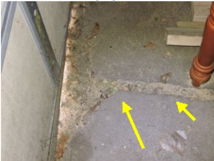
Example view - cracked/damaged garage floor
