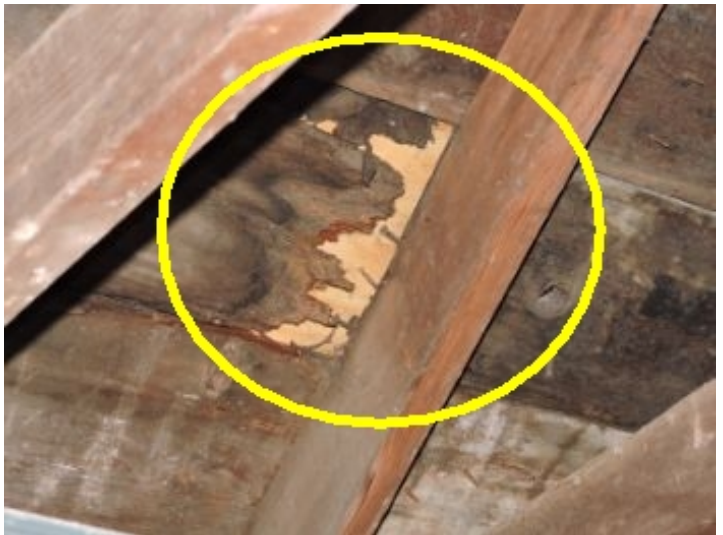
Example view - damage/prior repairs to board sheathing - garage
