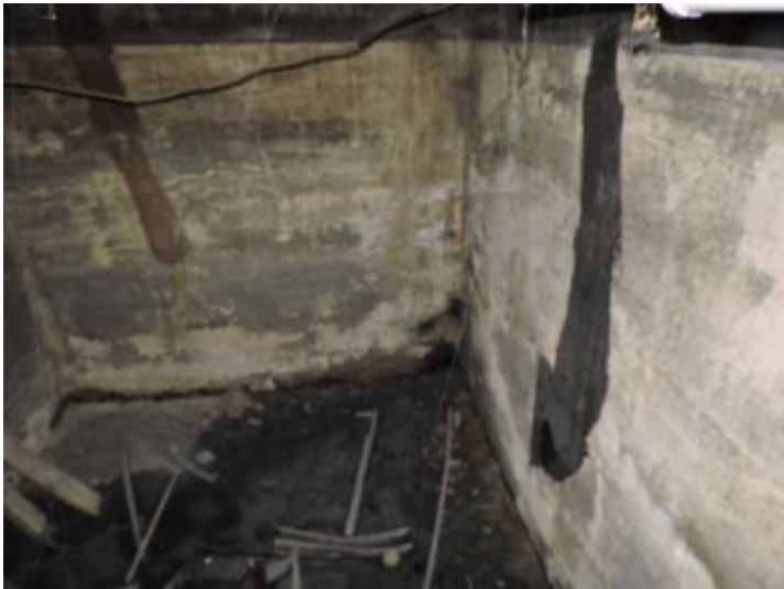
Example view - cistern
