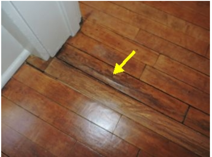
Example view - soft area at floor - foyer
