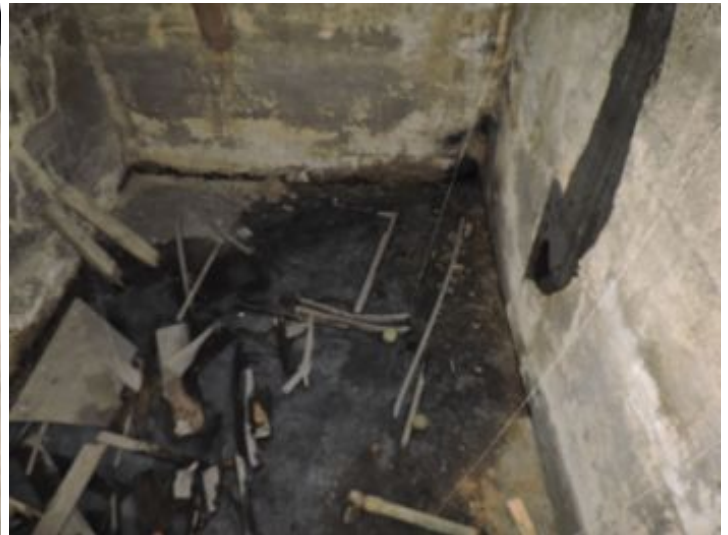
Example view - cistern
