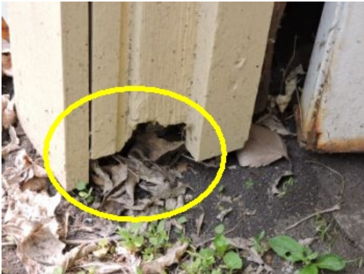
Example view - decay at garage passenger door frame
