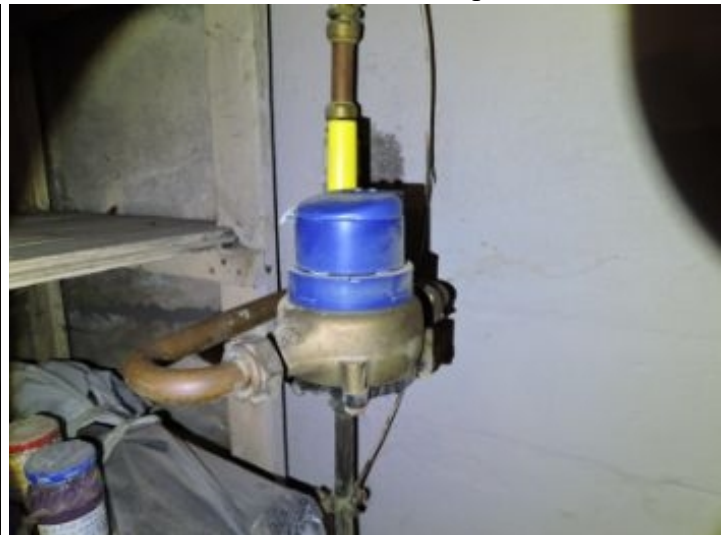
Example view - water meter
