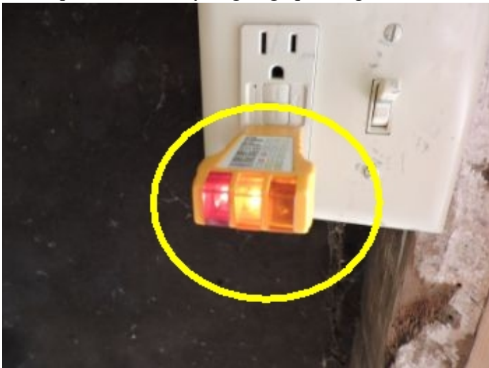
Example view - reversed polarity at garage GFCI outlet
