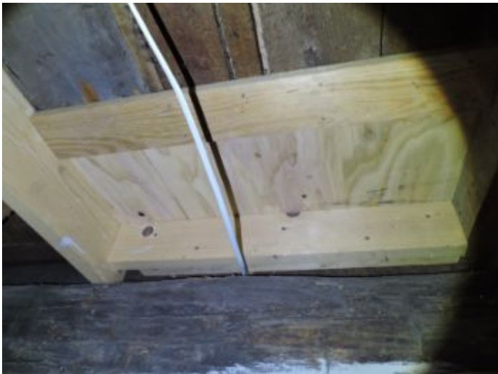
Example view - prior repairs to basement ceiling
